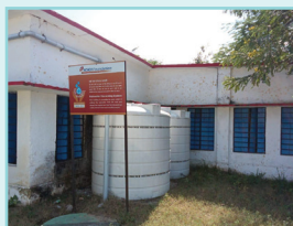
Rooftop rainwater harvesting
